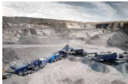
Combination of plants consisting of two cone crushers and two screen plants.
