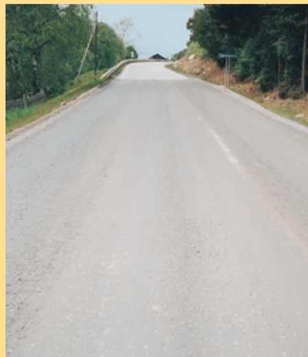
Vehicles can drive over the surface course bound with foamed bitumen before it is sealed.
