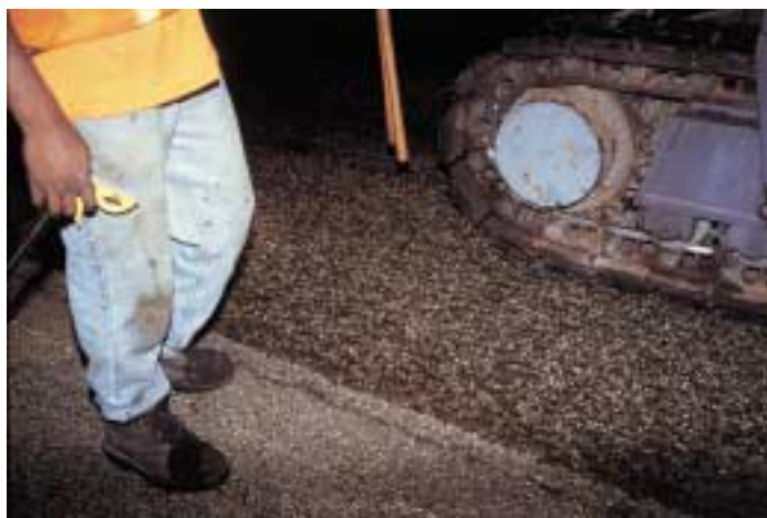
Fine, evenly milled surface means safer work zone and smoother final project
