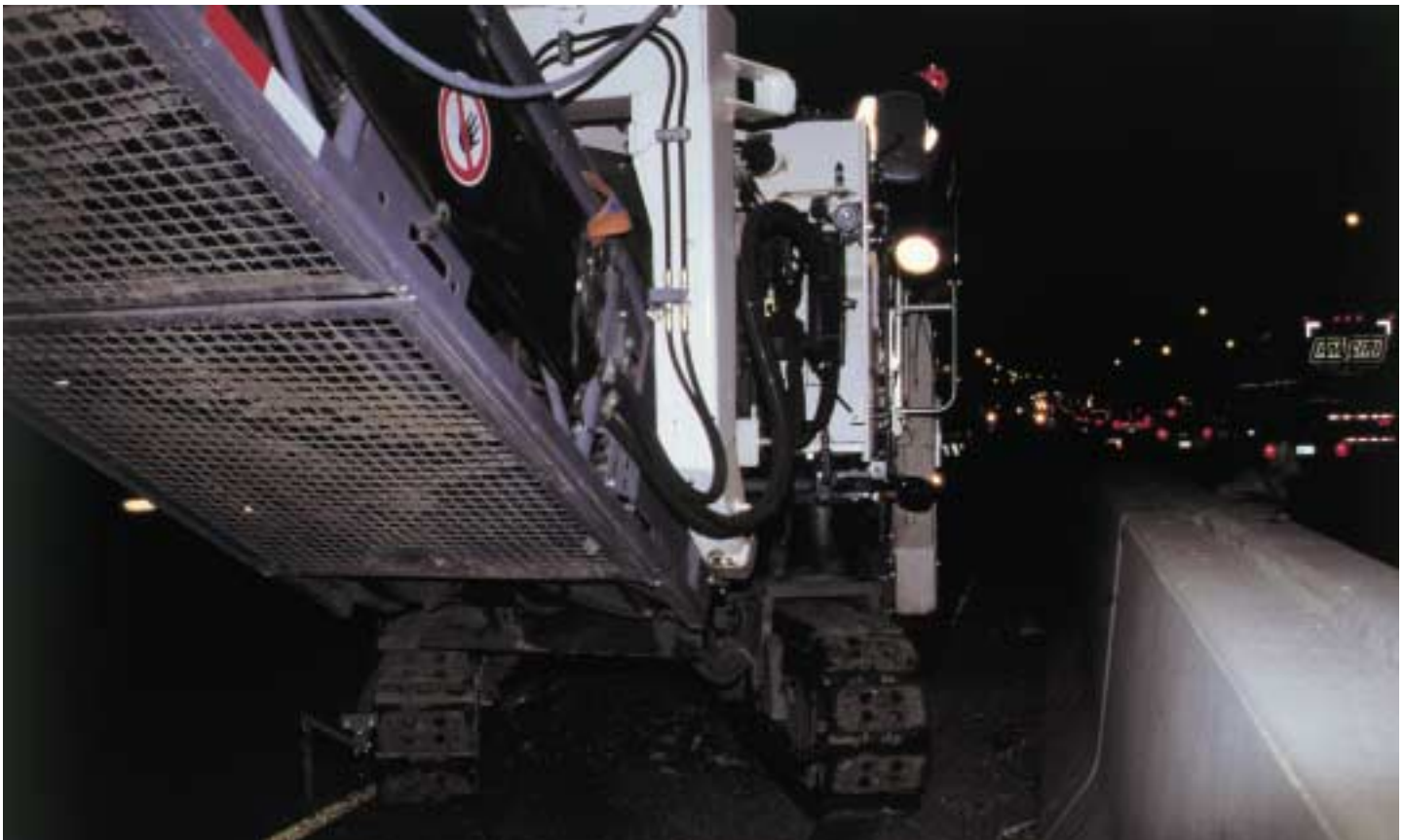
W 2100 maneuvers around iron inlet on elevated lanes
